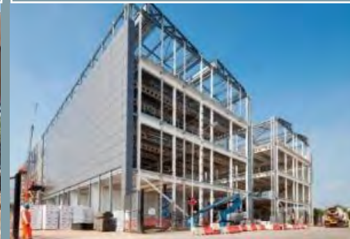
Data centre and other
