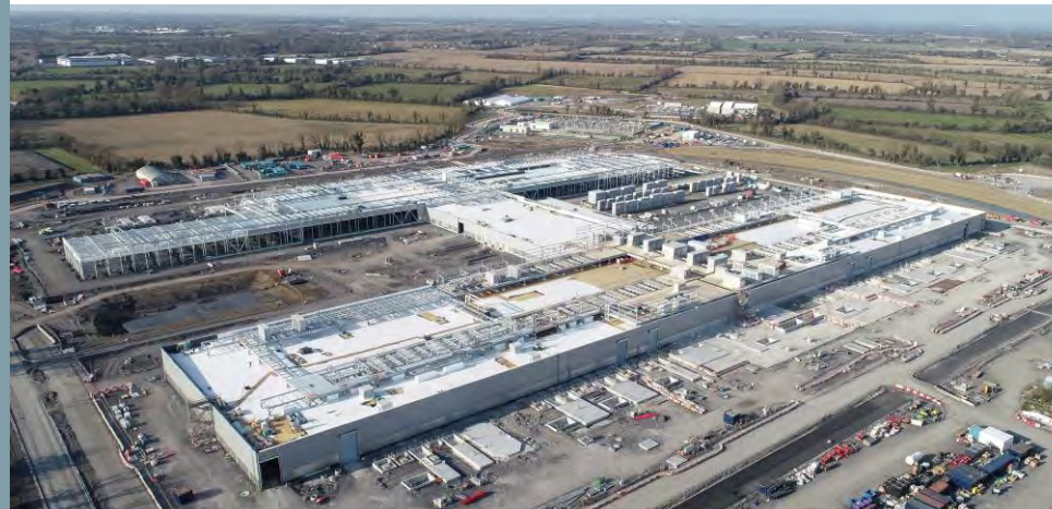
Data Centre Dublin
